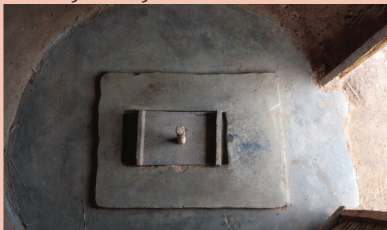
Inside Ceku's latrine. It has a washable floor and a tightfitting cover
